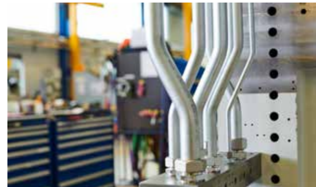
Pipework for the press with subsequent assembly of the infeed and outfeed
